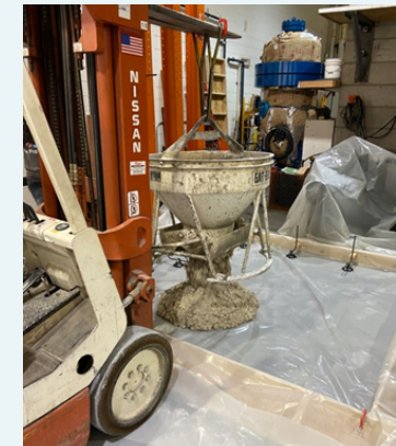
Carbon-negative concrete containing Minus Materials' biogenic limestone being poured, placed, and finished as part of a pilot demonstration in collaboration with Microsoft, the University of Colorado Boulder, and Boulder Ready-Mix Concrete.
